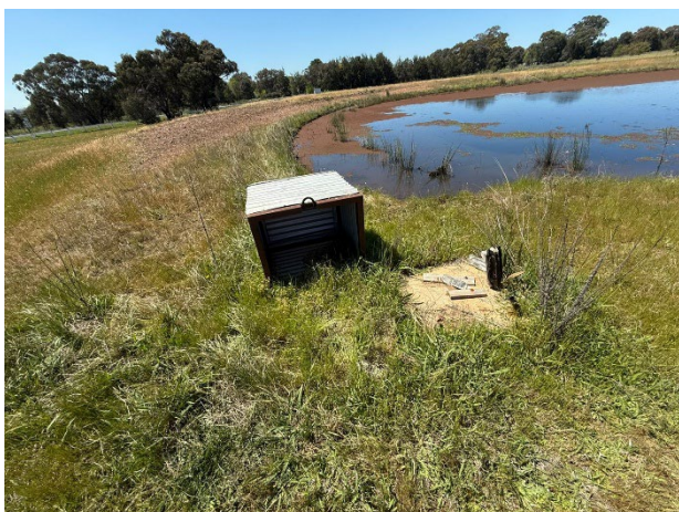
Image 3: Water pump infrastructure and pipes near the pond area; groundwater irrigation or livestock water access is likely.
